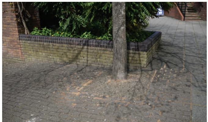
Existing tree roots damaging paving area
