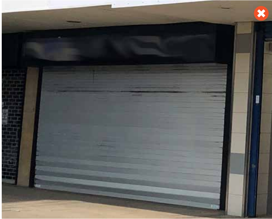
Figure 49. Closed type, external shutter unacceptable in any case
