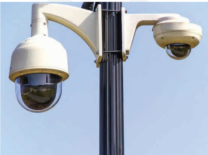
CCTV cameras mounted to existing lighting column
