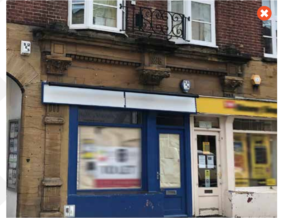
Figure 51. Alarm boxes haphazardly positioned on facade
