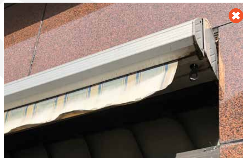
Figure 47. Blind box not well integrated with shopfront
