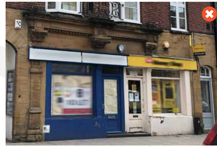
Figure 11. Fascia applied disregarding the building and obscuring pilasters
