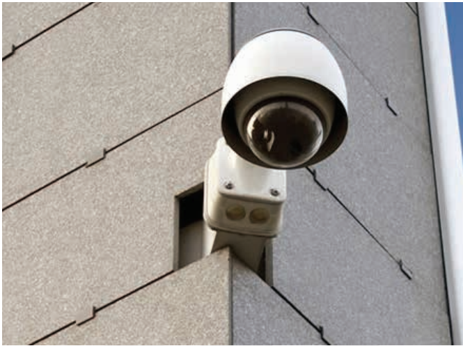
CCTV camera mounted to building
