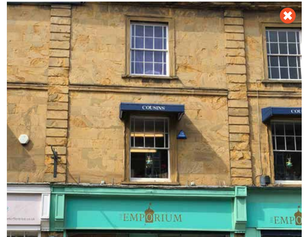
Figure 54. Alarm boxes haphazardly positioned on facade
